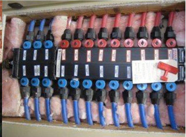
Photo 32 Water control manifold located in the garage utility room
