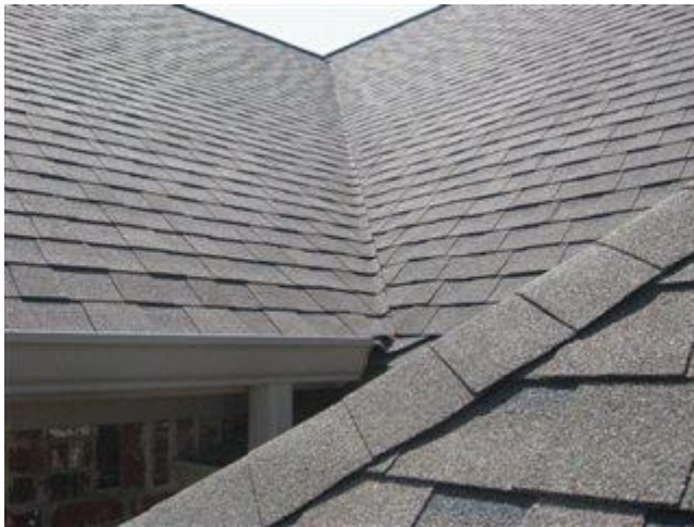
Photo 11 East side showing valley roofing method referred to as a cut valley
