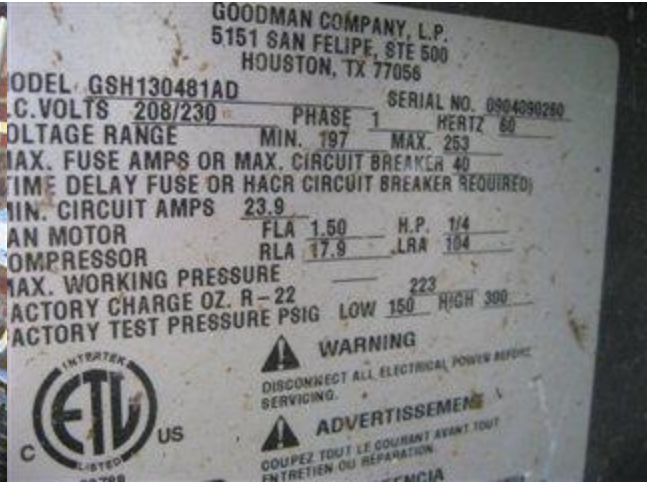
Photo 18 Data plate on outside AC compressor
