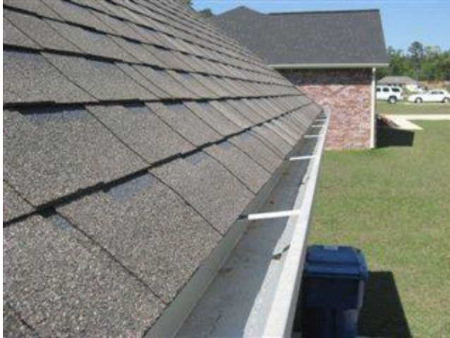
Photo 9 View of the east side showing architectural shingles with no defects noted and gutters that were clear with no debris or standing water
