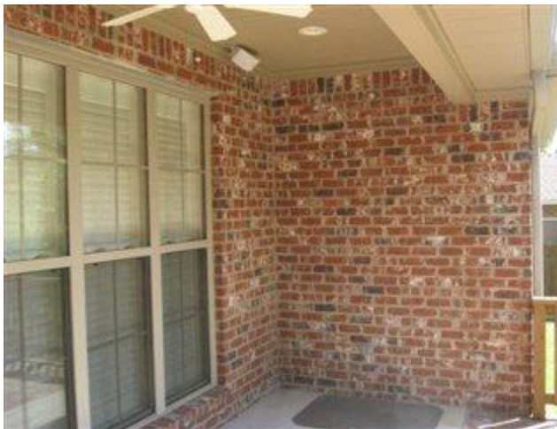
Photo 24 Recessed lights in rear porch ceiling
