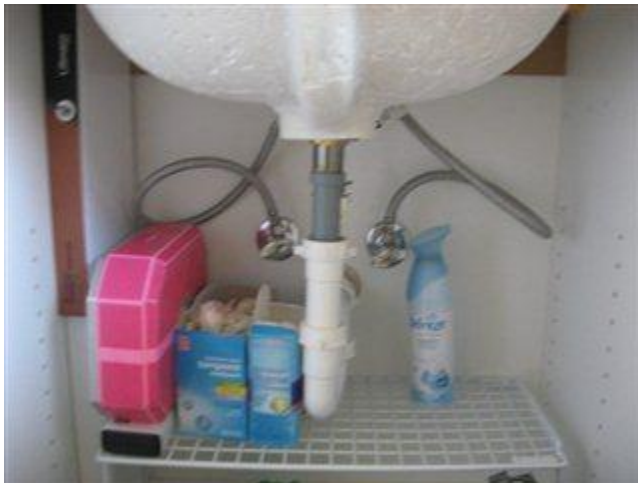
Photo 35 View of under sink areas in bathrooms with no sign of water leakage
