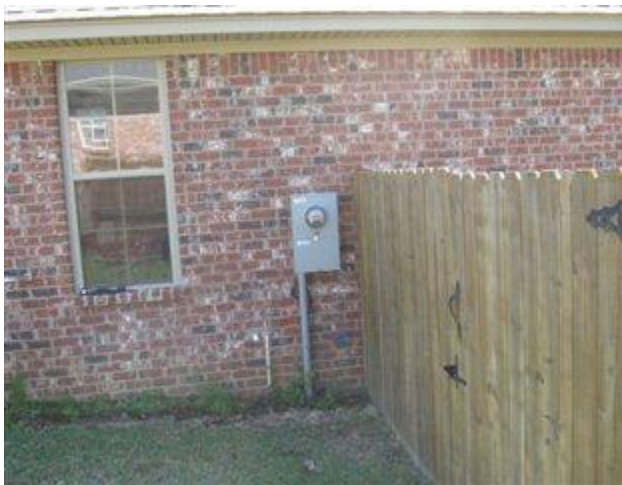
Photo 15 Electrical service and meter located on north wall
