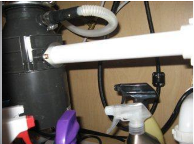
Photo 38 View of under sink area in kitchen with no sign of water leakage
