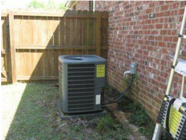
Photo 17 Outside AC compressor
