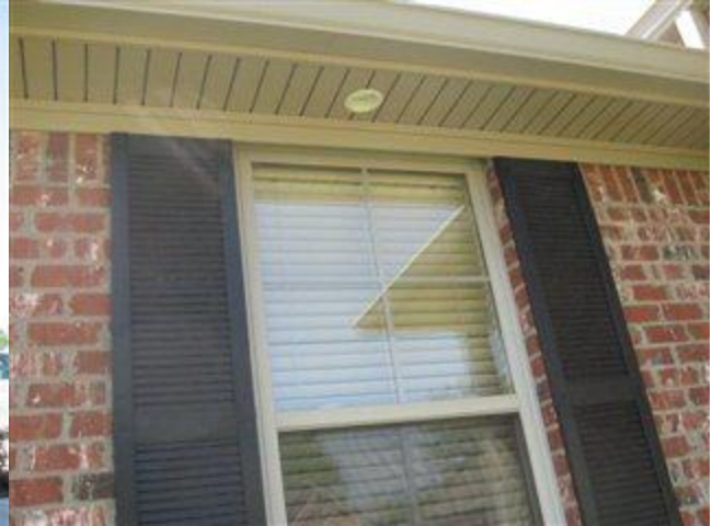
Photo 21 Recessed lights in front eave area
