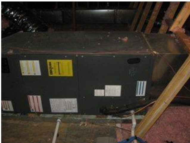
Photo 44 Horizontal furnace located in attic
