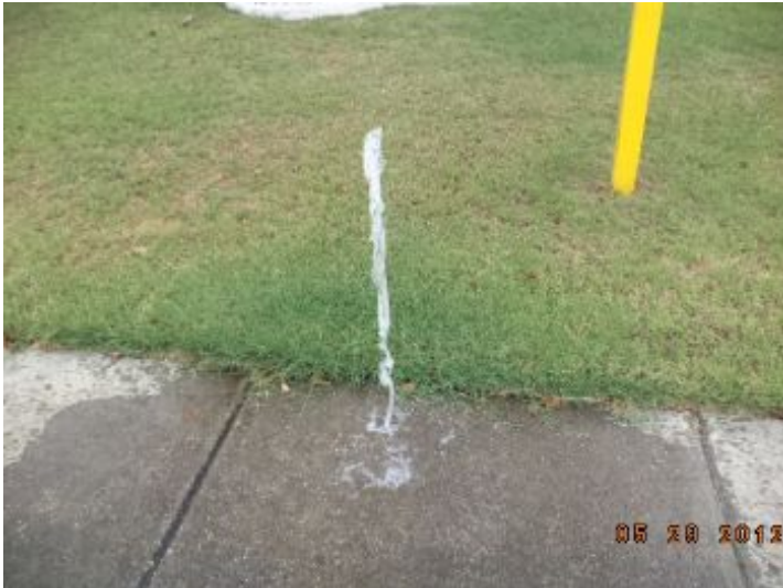
The inspector noted one broken head at the front left center. Zone 1
