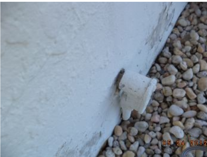
Seal around the electrical wire conduit at the front elevation, left side of the front door to prevent water penetration.
