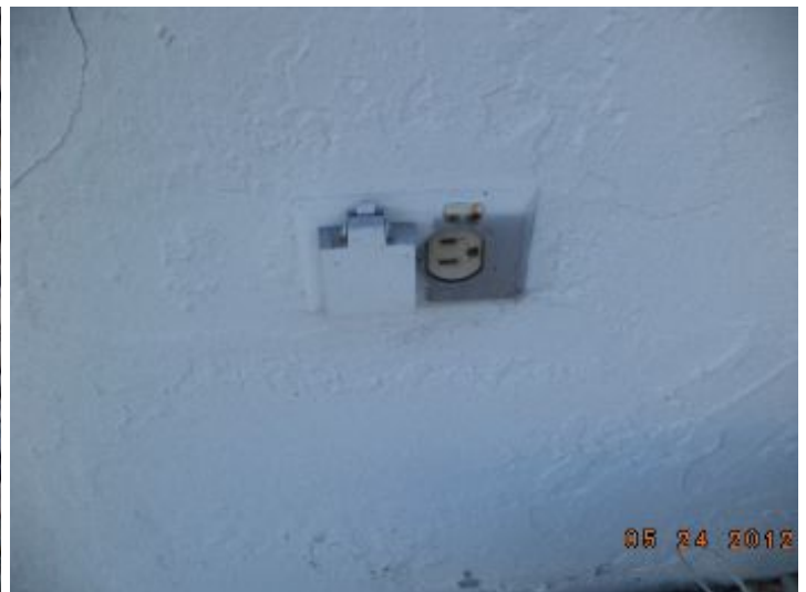
Replace the damaged waterproof cover on the left elevation outlet
