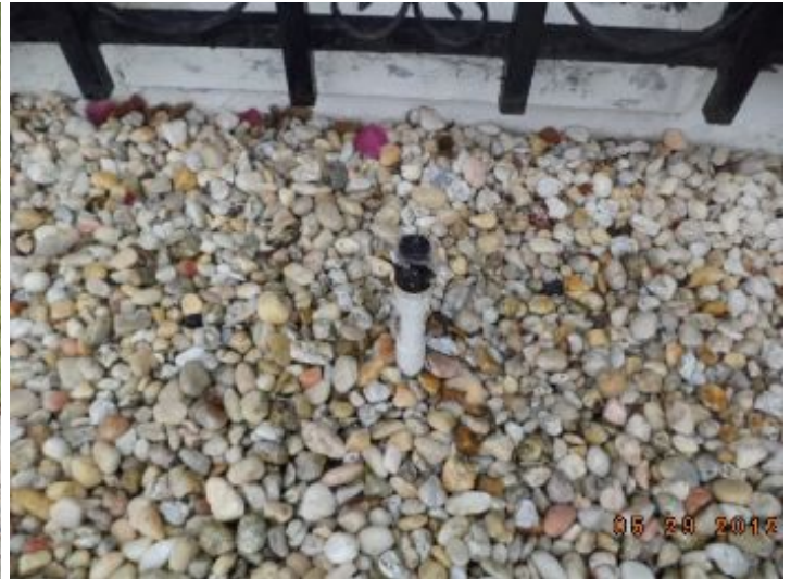
When operating zone 3, the last heads at the zone did not have enough pressure to operate properly. There were 19 heads on this zone, which is too many. I recommend a licensed landscape contractor check the system for proper water flow, sprinkler head repair and adjustment.
